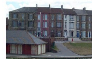
Newcomen Terrace maintains a substantial presence at the east end of the site, and refurbishment and improvement work is likely to be stimulated by new investment in the site.
